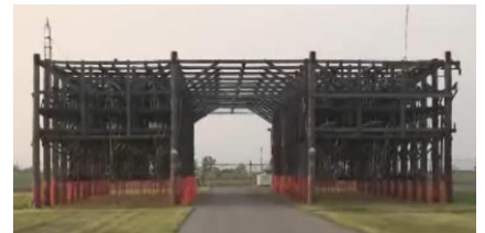
The Antenna switching Matrix.
