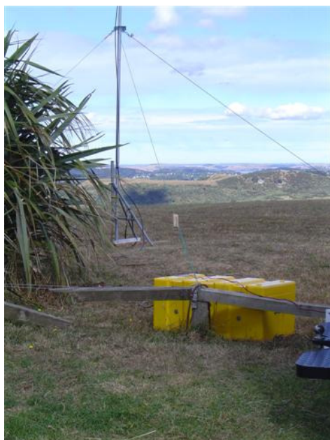
The WSRC Repeater
