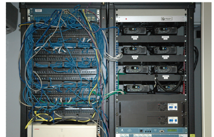
The radio racks in the communications room
