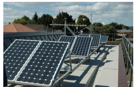
Solar Panels on the Roof
