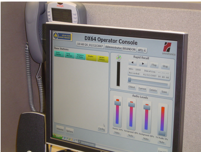
Radio Operators Console.
