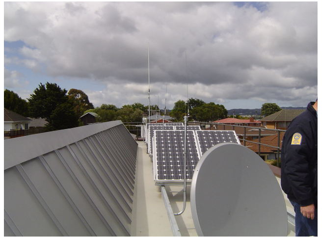
Solar Panels and VHF Antennae on the roof.
