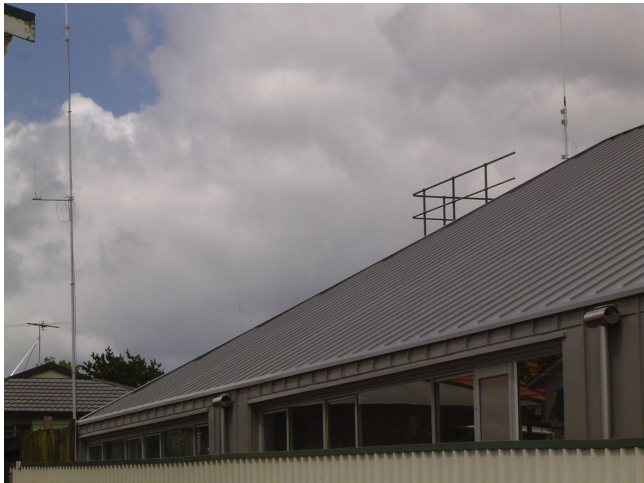
HF Antennae on the Western Side of the building.
