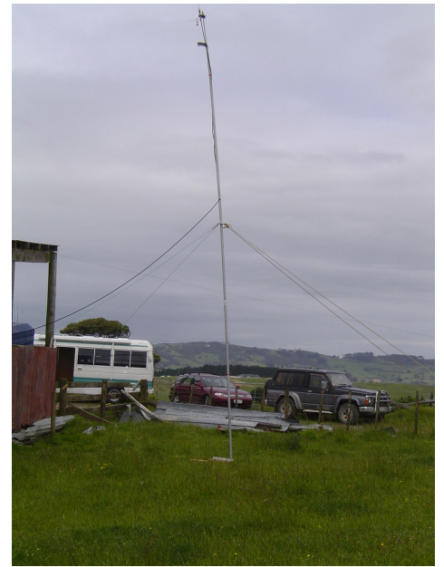
The Base Station Antenna
