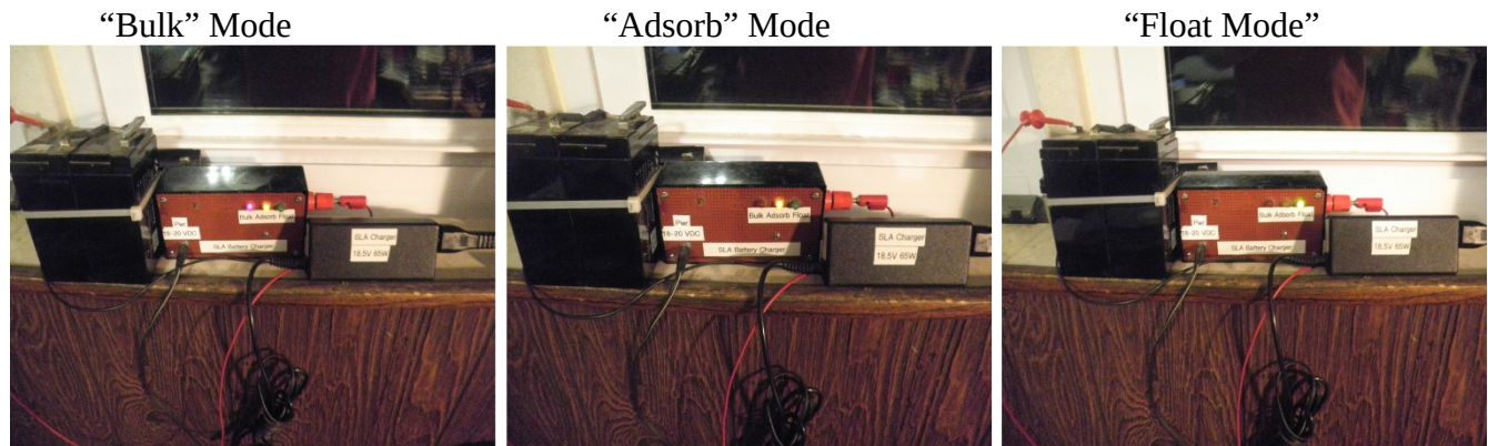
Figure 2: SLA Charger in use. Charging of an old SLA battery. Over 15 years old, but still takes a charge..
