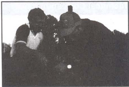
Figure 5—WA4UNZ and K4ZA work inside the large copper ground ring installing the feed system.
