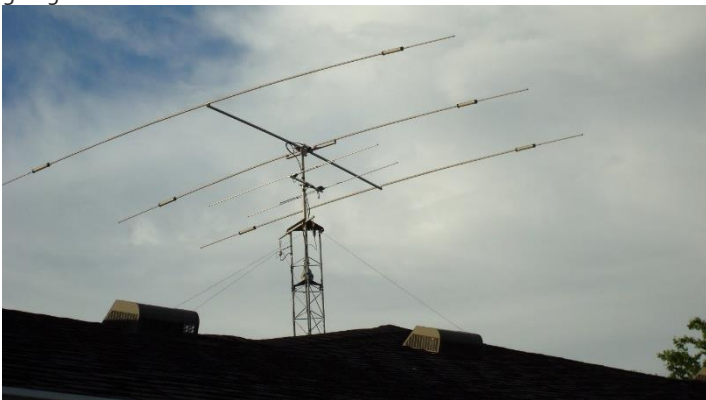
Diamond 502HB antenna mounted below HF tri-bander
