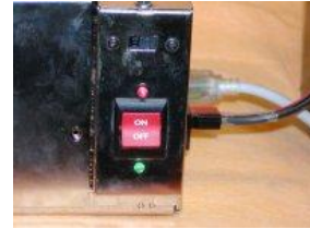
The original 110/220 switch is not used.
