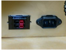
A PowerPole chassis connector is used to connect to the battery
