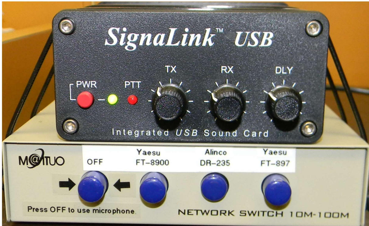
Figure 15. Signalink USB unit and network switch stack securely shelf-mounted at Station 17 Lomita with labels for three transceivers and instructions for operating microphone when configured for digital operations (Note that if/when the Bridgecom BCM-220 transceiver is issued to a given station to replace a failed or outdated Alinco DR-235, the label on this network switch can be modified appropriately.)
