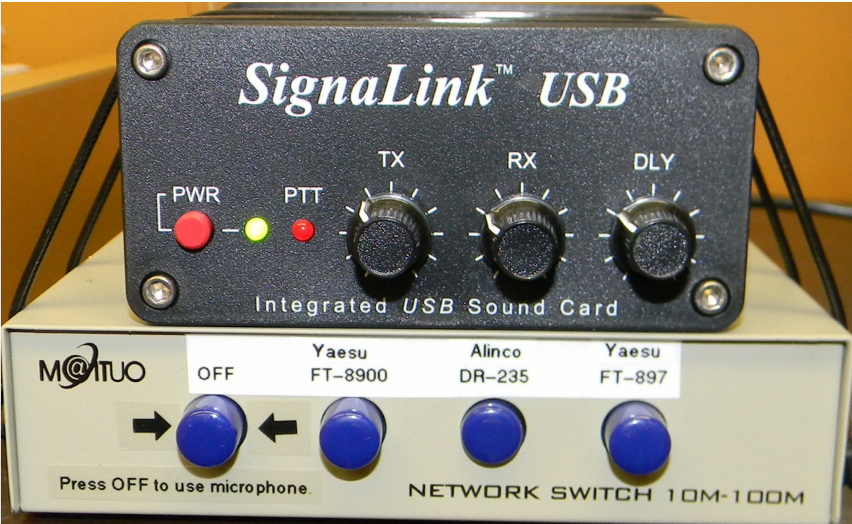
Figure 13. Signalink USB unit and network switch stack securely shelf-mounted at Station 17 Lomita with labels for three transceivers and instructions for operating microphone when configured for digital operations
