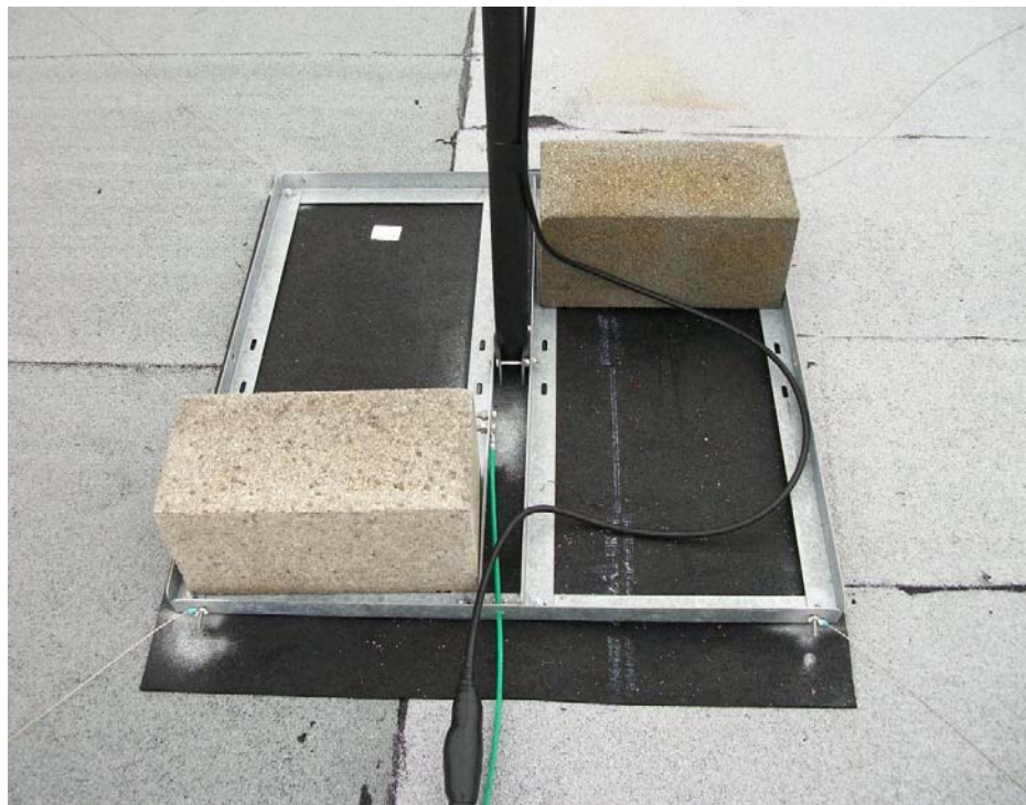
Figure 1-15 Center Mast Sled showing 4 ground radials and system ground.
