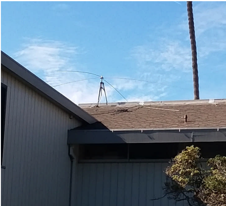
Figure 6. Damaged CB or other HF radio antenna atop the MDR Sheriff Station roof.
