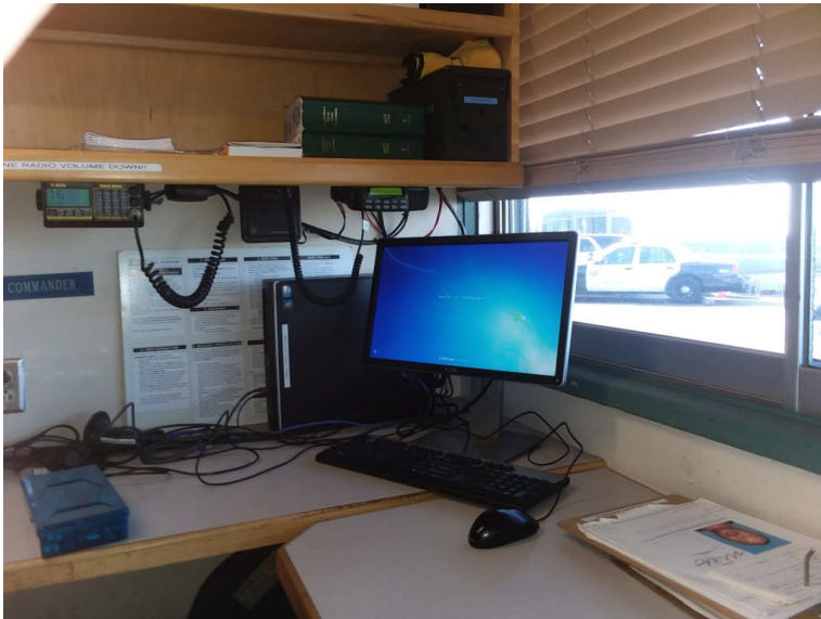
Figure 5. DCS radio and companion speaker location under shelf just behind and above computer monitor. Power supply is just off camera on the upper shelf and located roughly above the marine radio at the far left.
