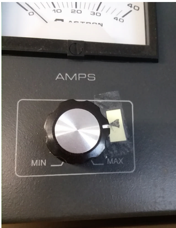
Figure 2. After locating the rotational position at which the “current limiting” AMPS control would enable full/desired output voltage of 13.8V without voltage scale-back, the control position was advanced a few more degrees clockwise and marked with a pointer to assure proper positioning in the future. This procedure was performed while drawing current with the radio in the high-power transmit mode.
