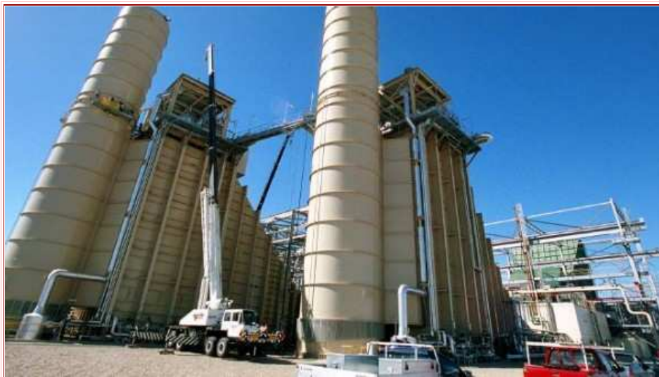
Photo 2 Pelican Point Combined Cycle Gas Turbine Power Station
