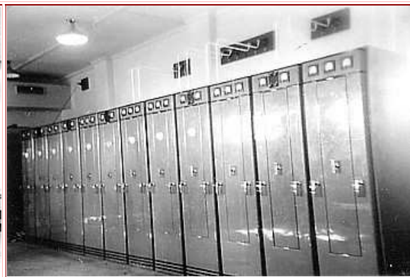
Leigh Creek AWA Multichannel Transmitter
