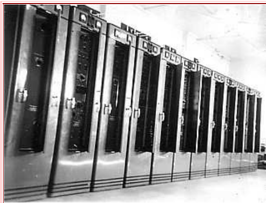
Leigh Creek AWA Multichannel Transmitter
