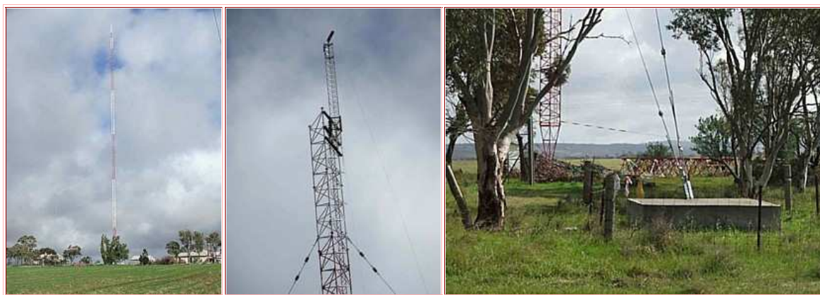
New 5PI cum 5CS Tower during erection in 2014 Photos by Ian Sutcliffe VK5IS
