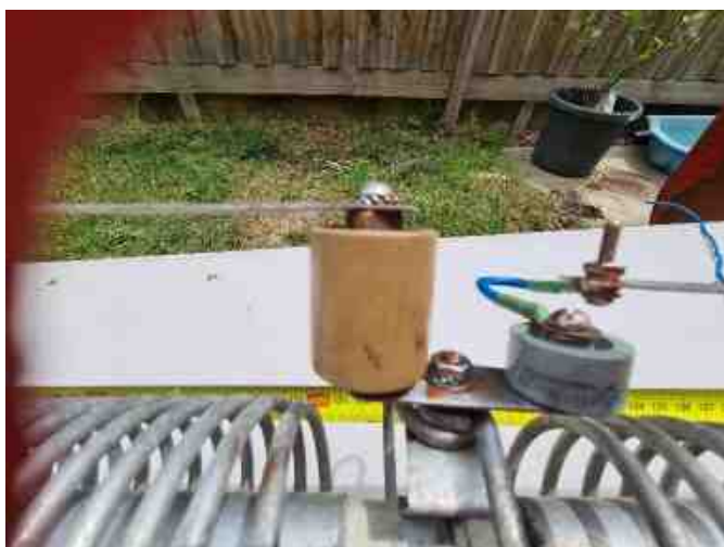
Replacement capacitor with stress relieve (right)
