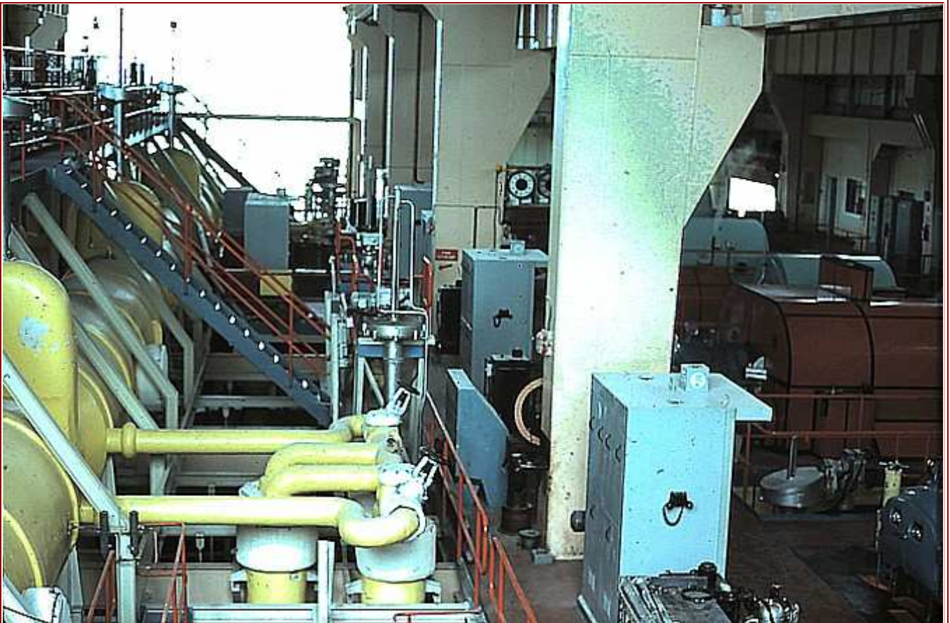
The Geothermal Power unit visited (On site photo by the Author)
