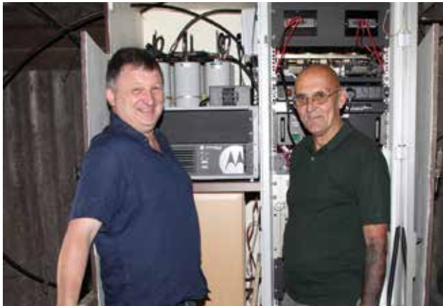
Michael, G1XCC and Mick, MOLEV with the new repeater. The cabinet also contains 23cm, 2m and 6m boxes.
