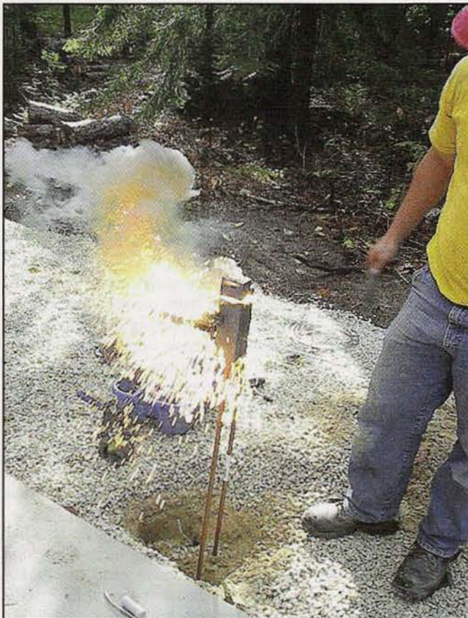
A spectacular shower of sparks as the Cadweld exothermic material burns, producing the weld between a #2 copper wire and a 5/8-inch copper-clad ground rod. The black color graphite mold containing the molten weld metal is clearly seen.
