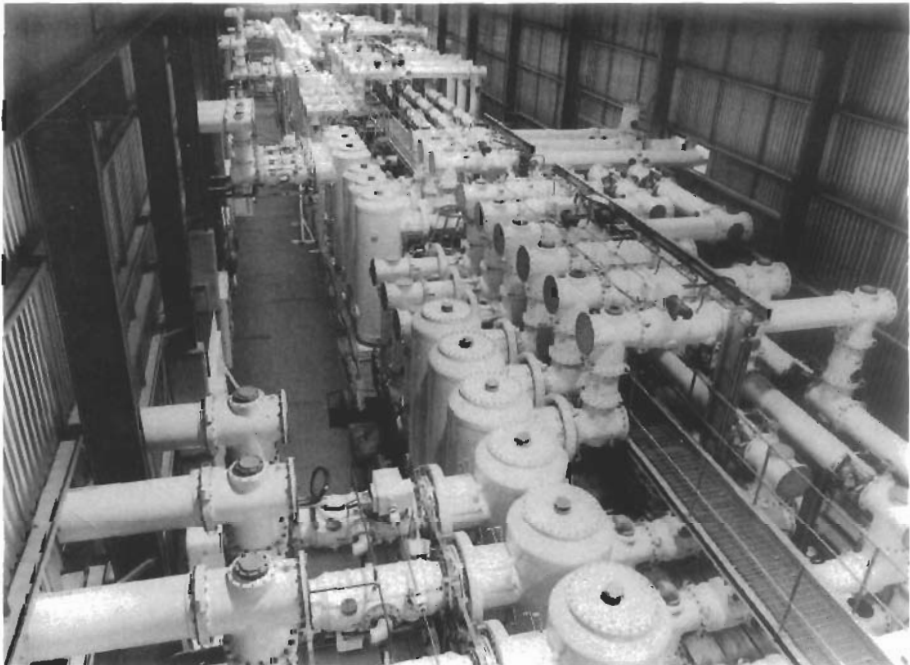
Fig. 7.27 Example of a GIS substation
