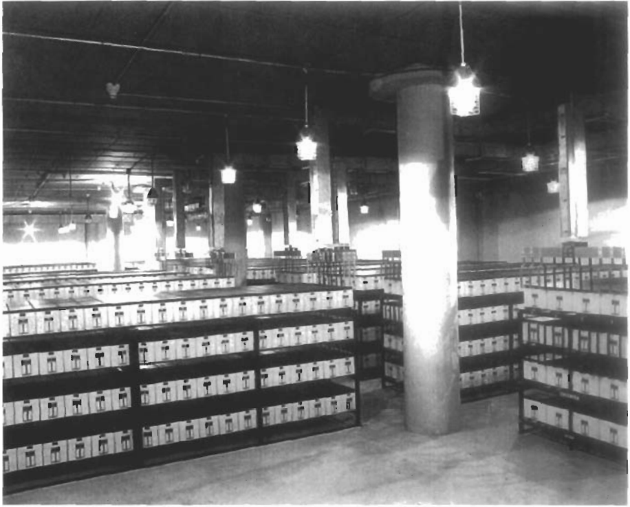
Fig. 12.29 Typical battery installation (courtesy of Invensys)
