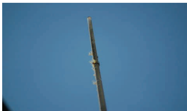
Take a look at Mauna Kapu antenna with moss and rust.
