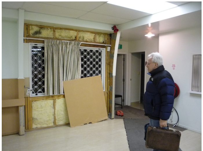
Dave ZL1MR looking at the work in progress with the water damage
