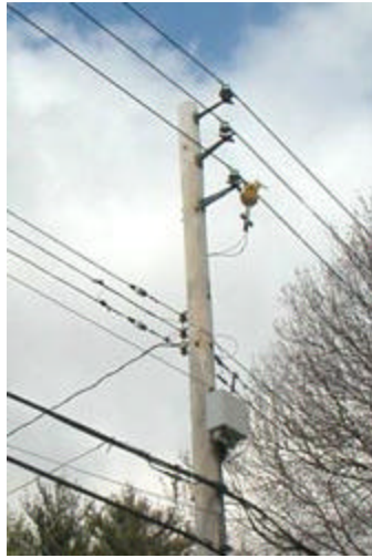
An Ambient BPL power-line connection in Briarcliff Manor. The yellow object is a tap off the medium-voltage primary. The gray cabinet holds the electronics. [Alan Crosswell, N2YGK, Photo]
