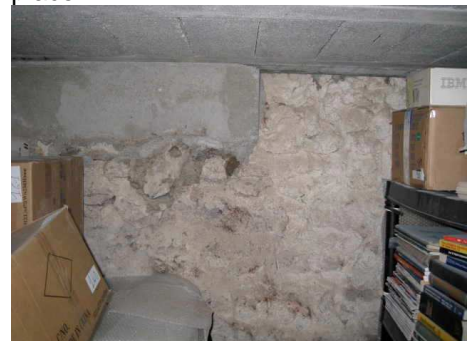
Basement side with no hole
