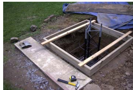
All this talk about the tower at W2CGX... Here's what the "hole" looks like before cement is added.
