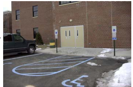
New loading doors complete with built-in ramp, and it's close to the vendor area!
