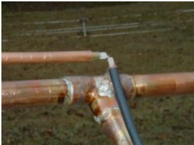
Another closeup of the feed point on Van's antenna. He hadn't mounted a connector at this point but had connected the feedline to do preliminary adjustments. Nice job Van!
