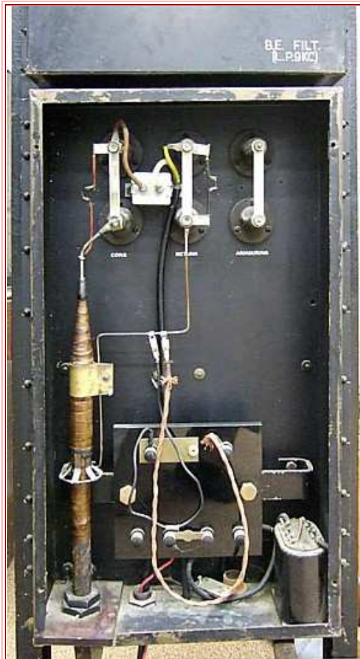
Cable Termination Cabinet, Apollo Bay
