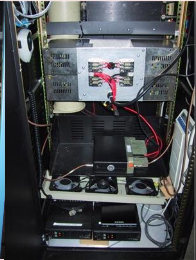
McKinney, Tx 145.350 VHF Repeater
