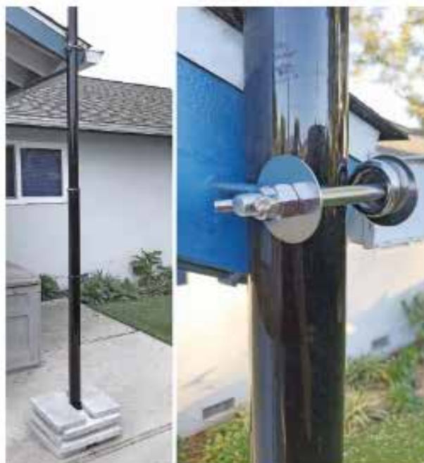
Figure 4 — What the mast looks like once it's mounted to the eaves. Note the stack of heavy patio bricks holding the mast in place.
