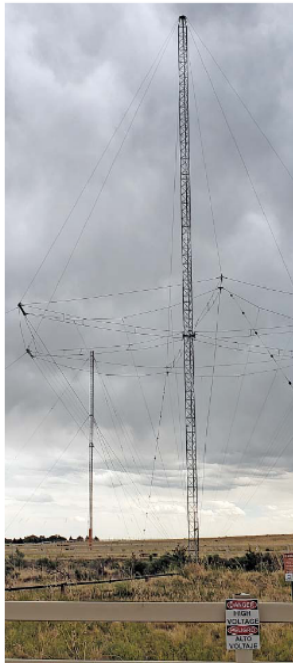
Figure 1 — The antenna in the foreground is a standby broadband antenna with an inverted cone design. It can operate at any of the WWV frequencies from 2.5 to 25 MHz. The primary 5 MHz antenna is in the background.
