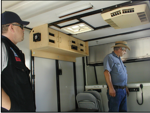
The Starter for the Generator is Right Here...
