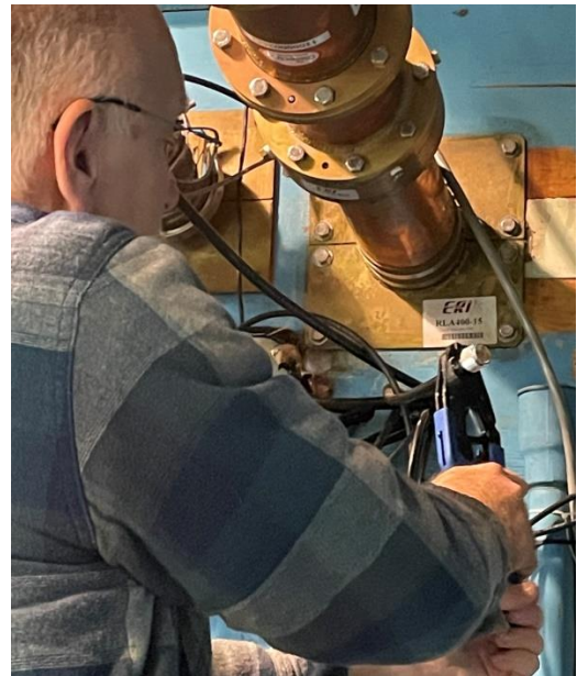
And crimping the new connector into place.
