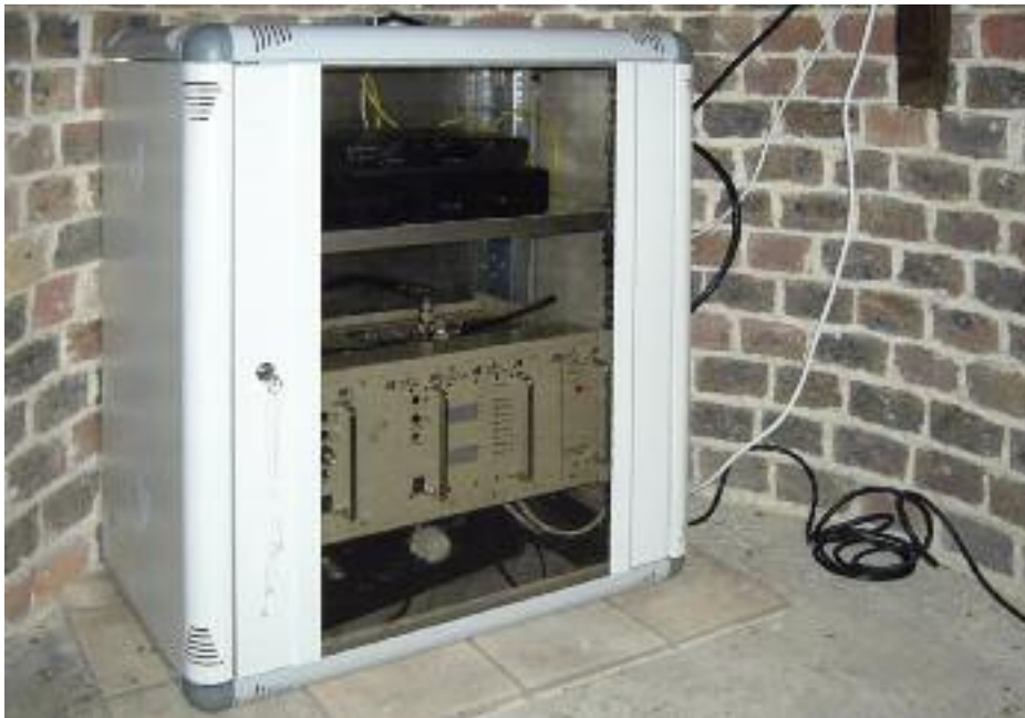
The homebrew D-Star node lives in a professional-looking rack enclosure in the tower of St. Leonard's Church, Turners Hill.
