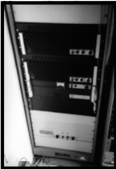
Some equipment at Barkway
