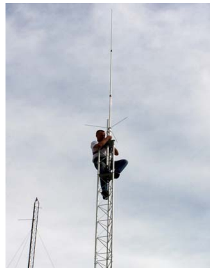
As a result, the first antenna is now in place at the QRM Room
